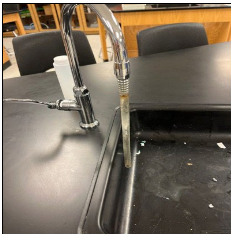
View of potential DWO and sample 04-01-105-CF-P-16 (No sample taken. Outlet was offline.)
